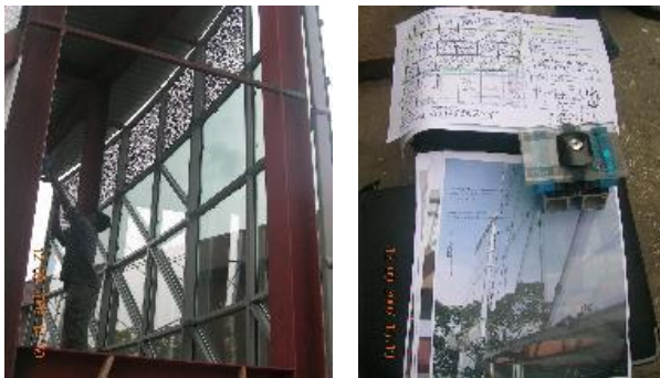
Figure 161: VMU Of Monocoque Frame And Glass Condition
