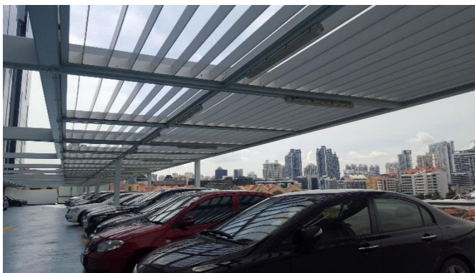
Figure 102: A Basic Brise Soleil As Shading Device For Vehicles At The Outdoor Carpark Of CENTRAL Mall In Singapore. (Courtesy: Patricia Collera)
