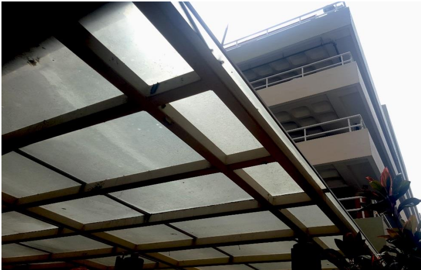
Figure 36 Canopy Laminated Glass With Frit Coating. (Courtesy: AgFacadesign & G FACADESIGN Pte Ltd).
