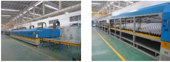
Figures 73 And 74: Heat Oven And Quenching Compartment Of Tempering Line
